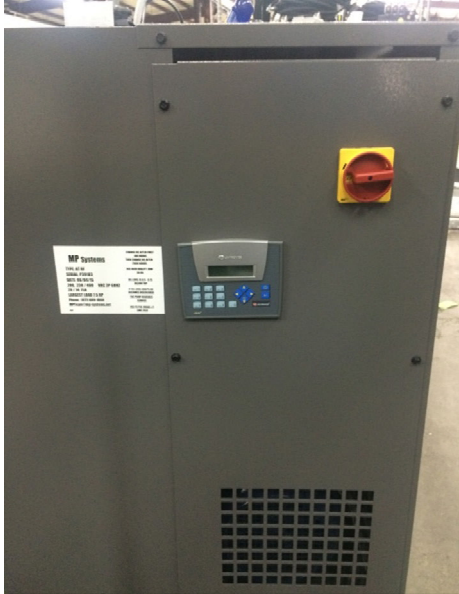
Power off R Series. Remove electrical panel door.
